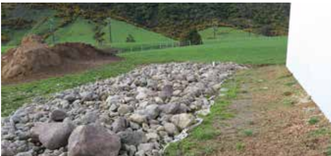
DETAIL: The soak hole for the run-off from the barn floor. The total wintering barn cost of $280,000 included construction, internal fit-out, concrete feeding strip and drainage. Photo: Tony Leggett
