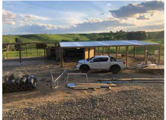
REVAMP: A deer handling facility was adapted from an old milking shed, taking advantage of the established concrete floor and roof, electricity for freezer storage and lighting, plus the roading for trucks to offload or load deer.
